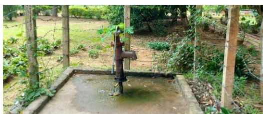
Fig.2 :Bore well in the Campus
