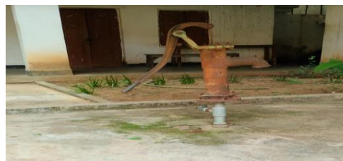
Fig3:Bore well in the Hostel
