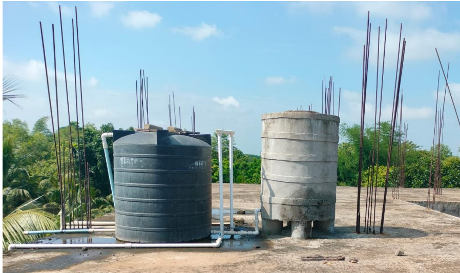
Sintex Tanks of Hostel
