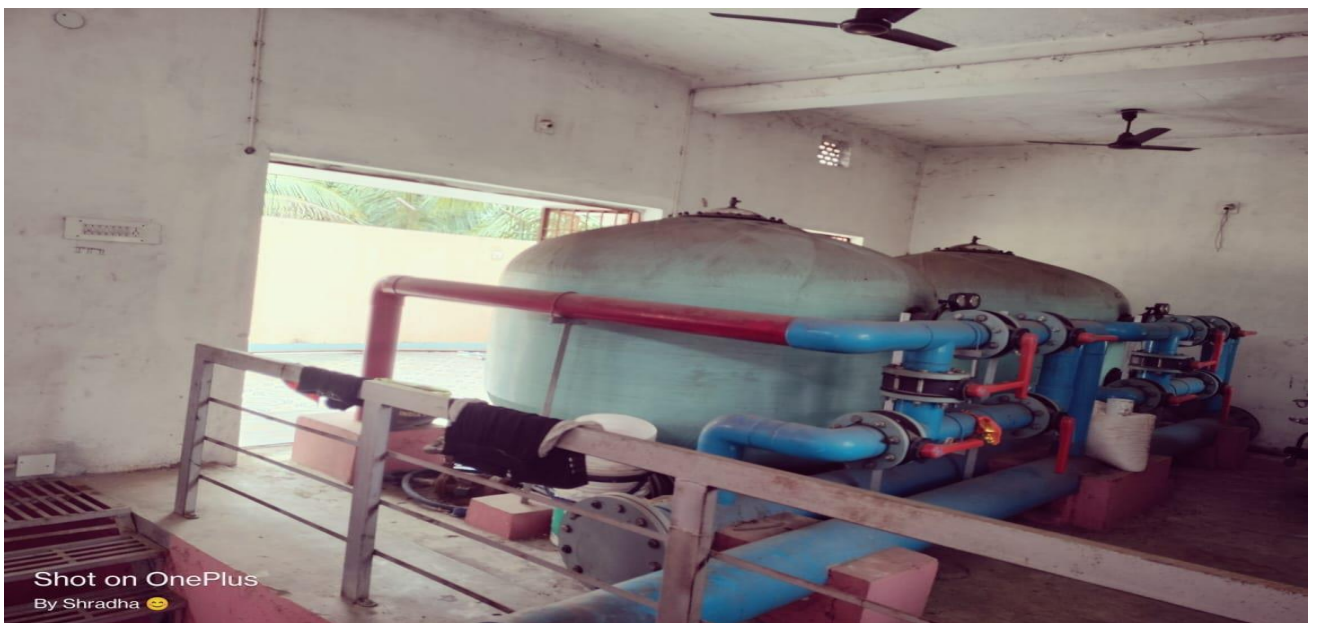
Water Filtration Unit
