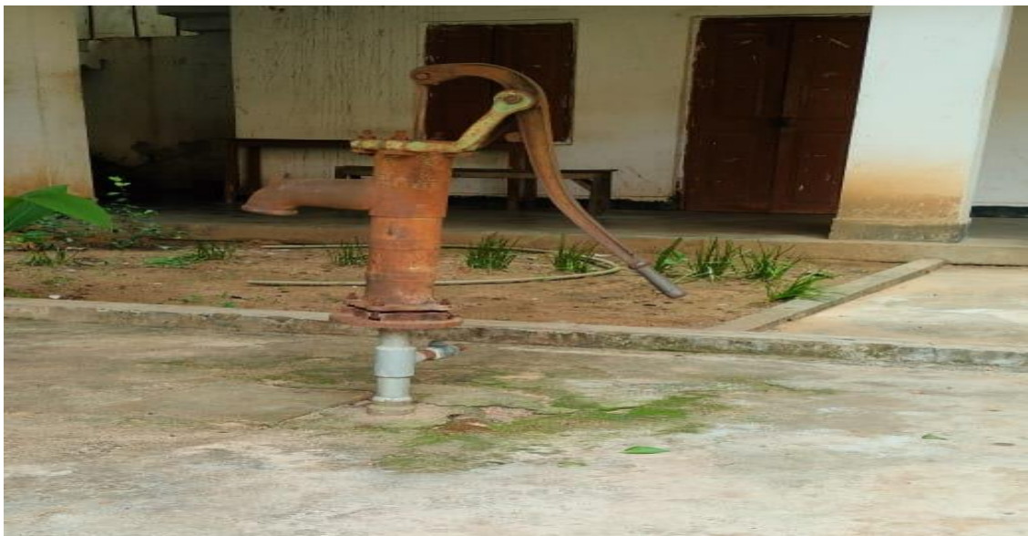
Bore well in the Hostel
