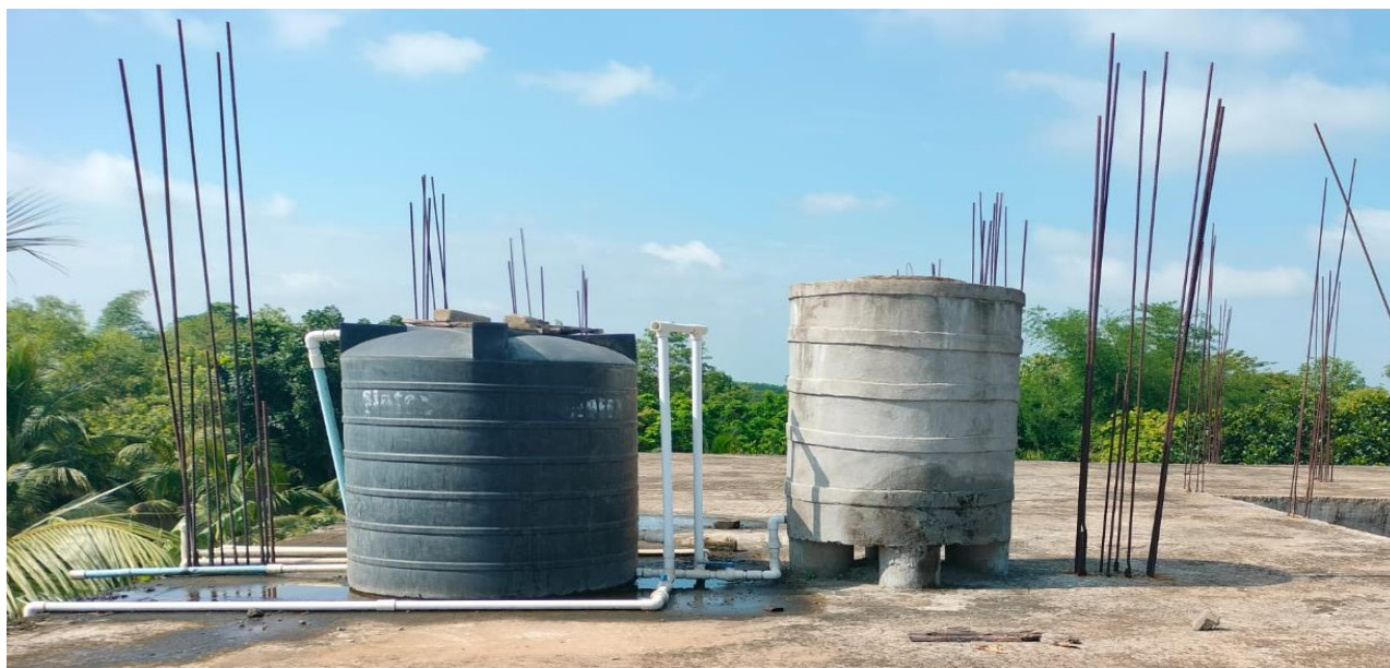
Sintex Tanks of Hostel
