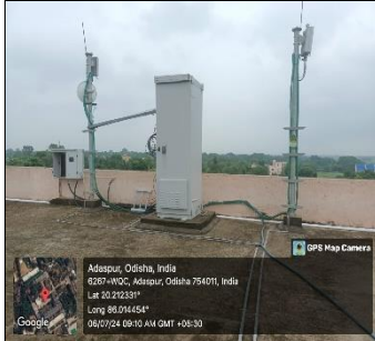
INTERNET FACILITY TOWER
